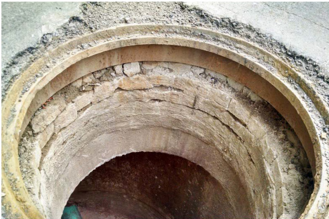
Representative manhole in need of repair.
